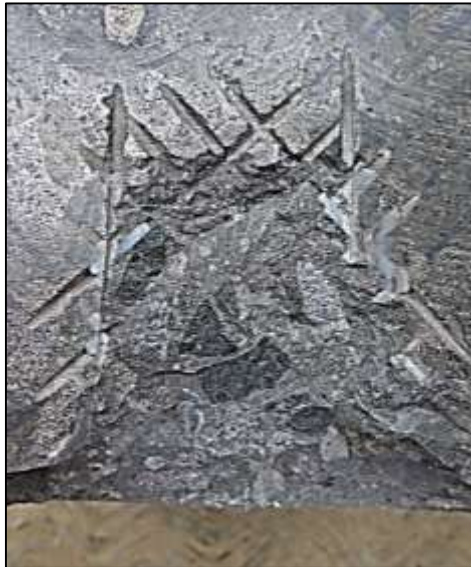
Concrete shear failure
